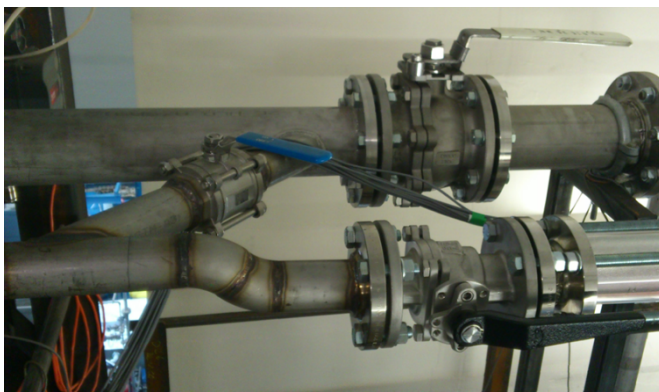
Fig. 60: Bridge valve between the 4" line and the 2" line
