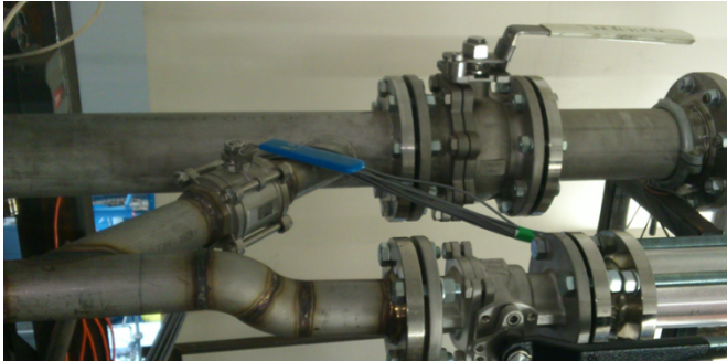
Fig. 26: Bridge valve between the 4" line and the 2" line
