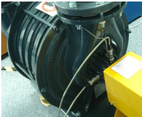
Fig. 112: Compressor driven end
