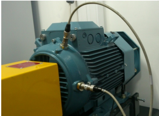
Fig. 110: Motor casing accelerometers
