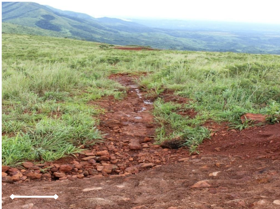
Figure 3.3. Rill and gully formation observed in the Simandou landscapes adjacent to a mine-site haul road (2cm = 1m)
