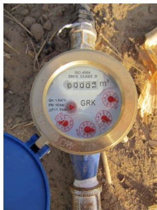
Picture 3.5 Water meter installed at each field
