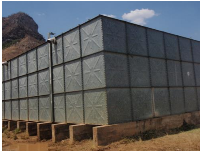
Figure 3: Water tanks supplied by BWB
