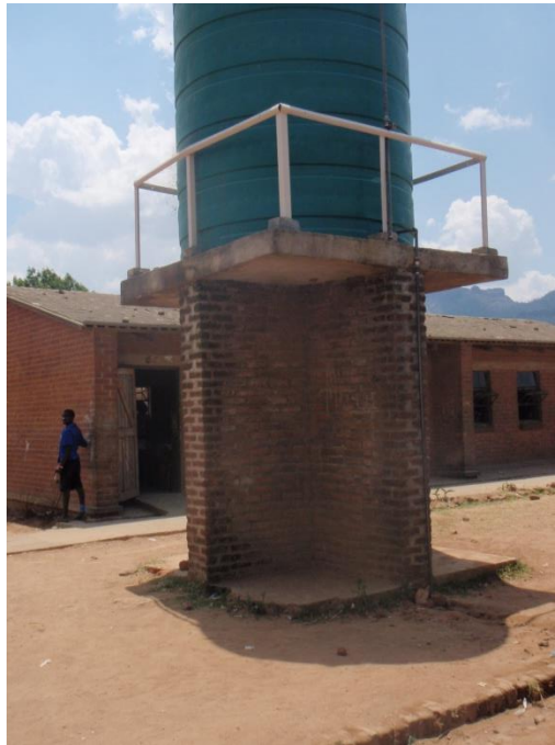
Figure 4: Water storage tank at local school
