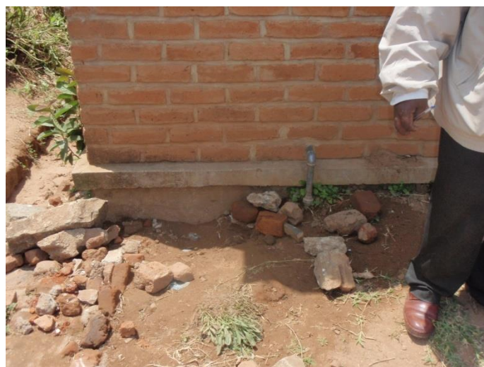
Figure 5: Pipe work stolen at local school
