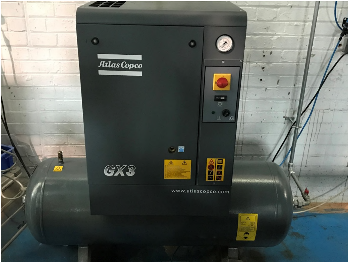
Figure A.1-5 Pneumatic valve service compressor (PVSC)
