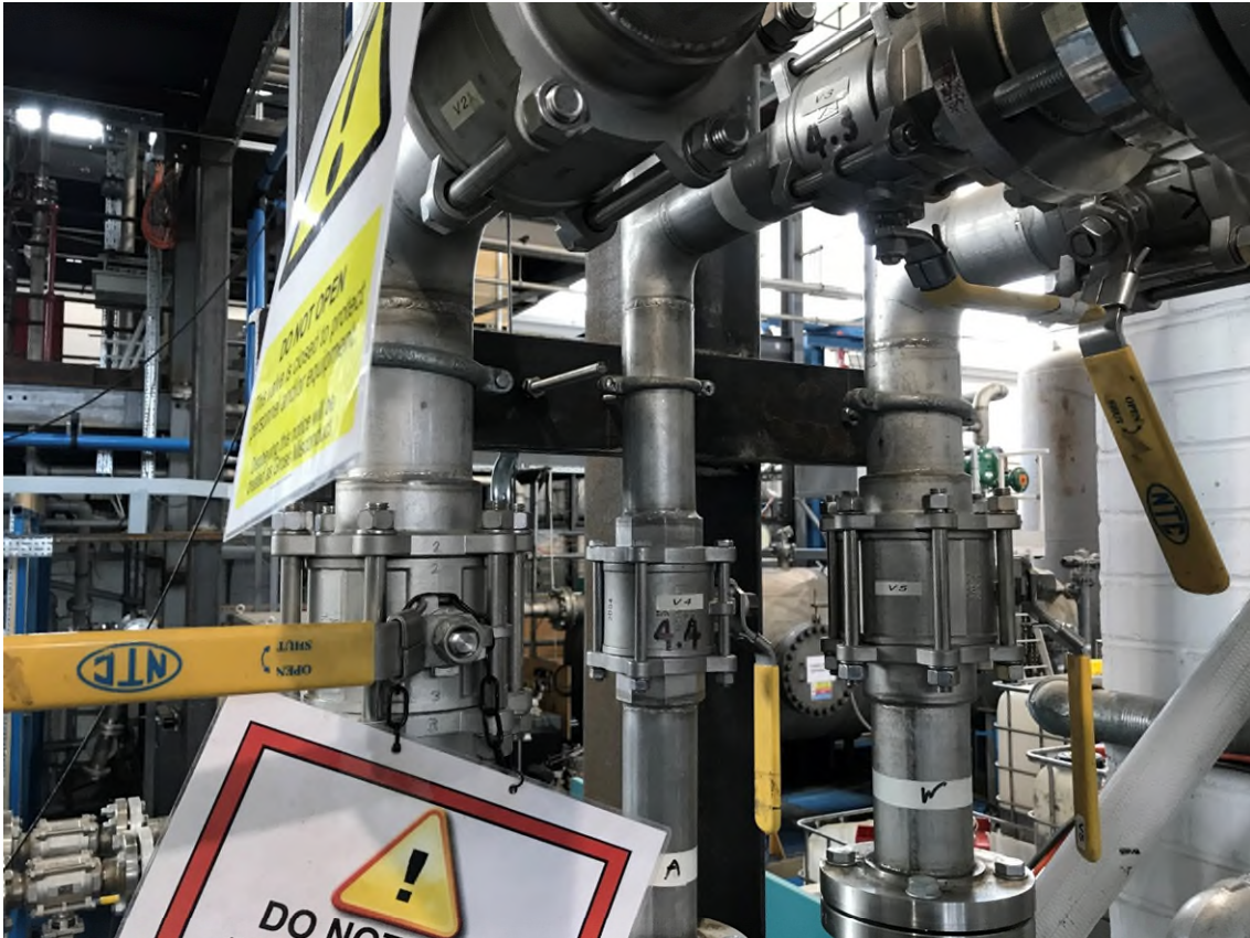
Figure A.3-1 Some valves in valve manifold section
