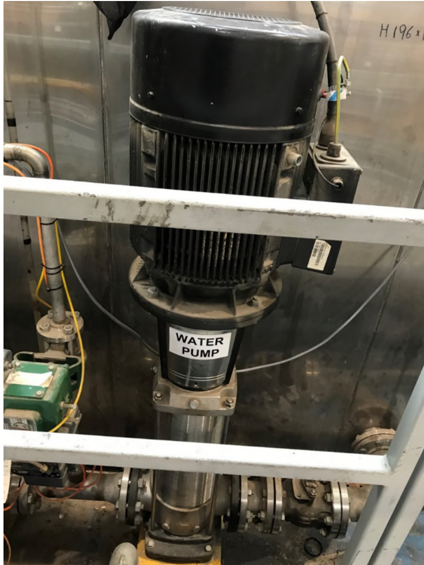
Figure A.1-6 Water pump
