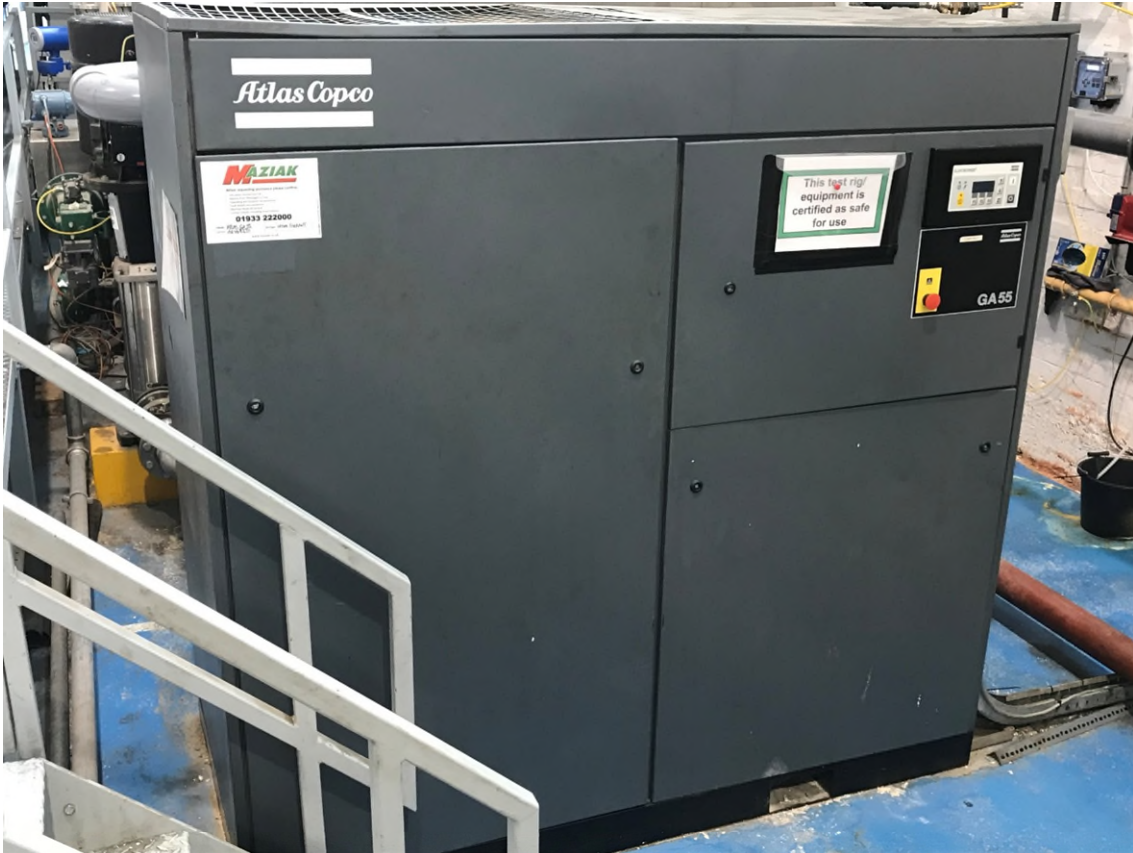
Figure A.1-1 Air Compressor
