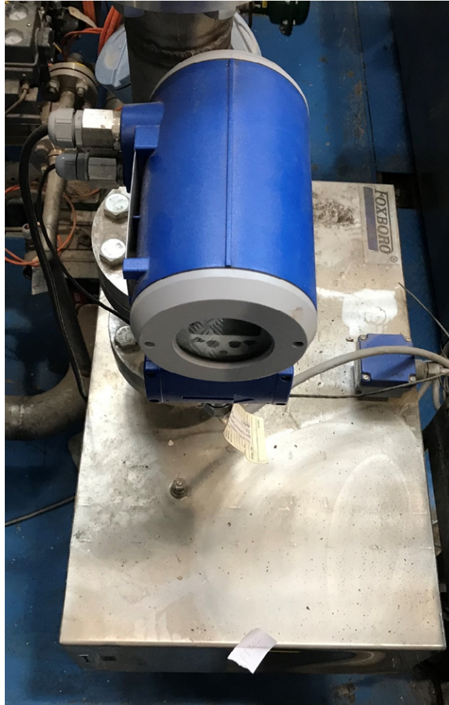
Figure A.2-1 Flow meter
