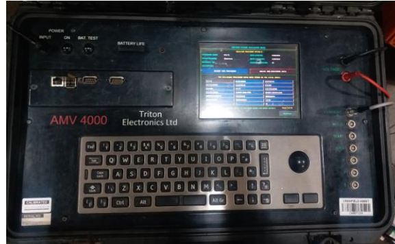
Figure 4-7 Arc monitoring system used for arc characterisation
