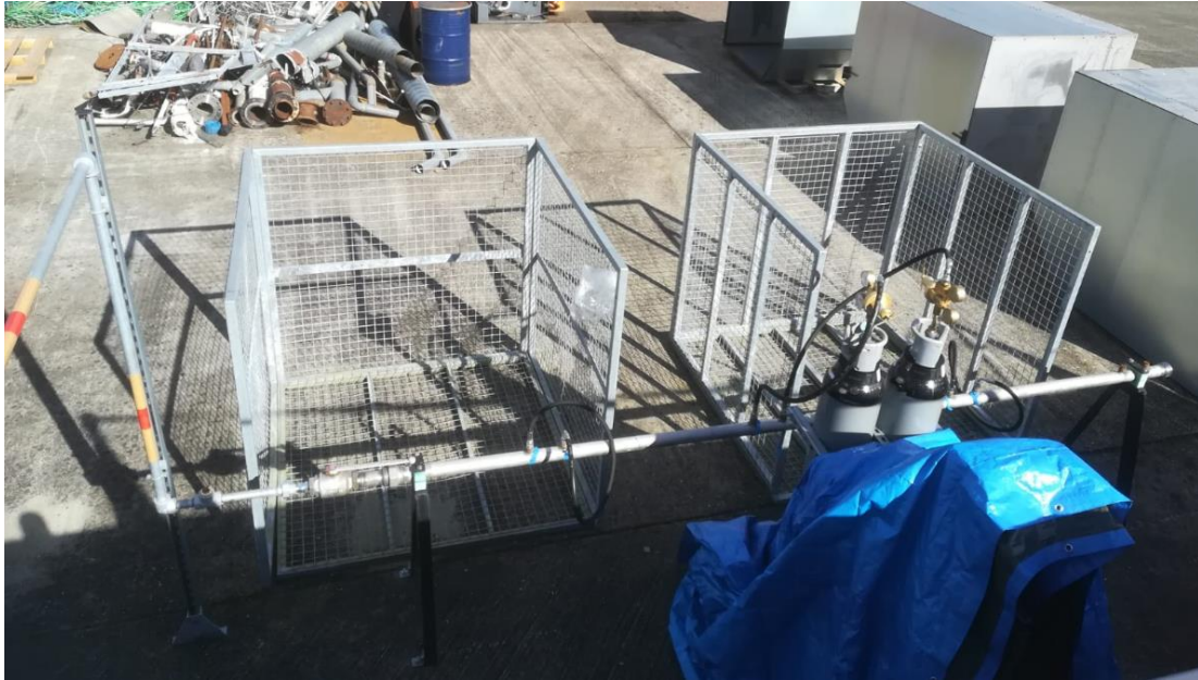
Figure 106 - Nitrogen storage cylinders and distribution network
