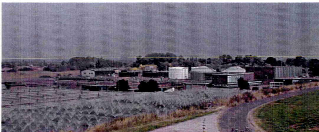
Figure 1.4. General site view of Wanlip STW, showing banks of trickling filters (front left), activated sludge tanks (rear left) and large circular digesters (right).
