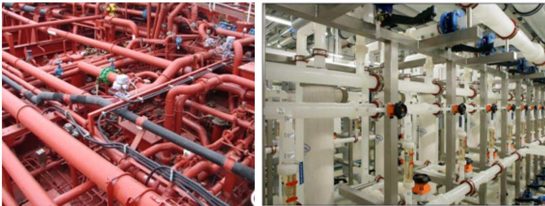
(a) piping system of a chemical tanker
