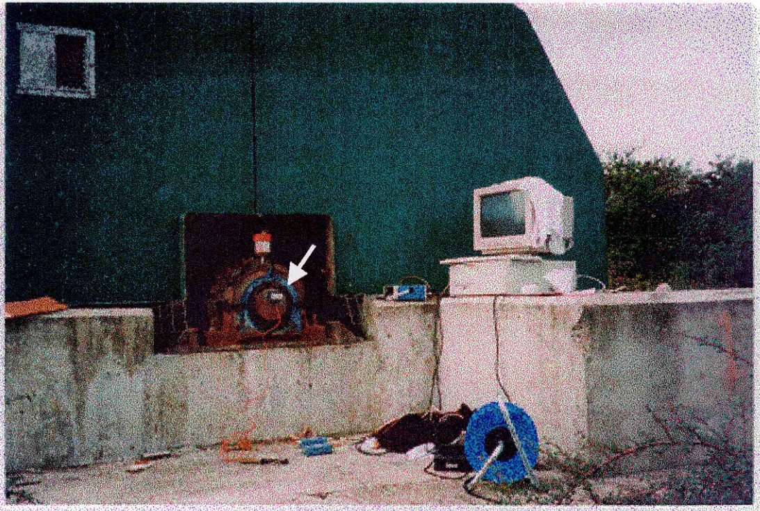
Photograph 8.1 Placement of sensor on stub shaft, STW Illmington
