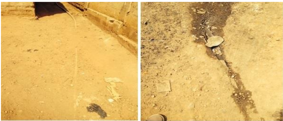
Figure 4-1 Exposed inch pipeline and burst inch pipeline
