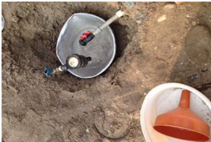
Figure 4-9 Hole dug in the ground to access water because of low pressure in the distribution system
