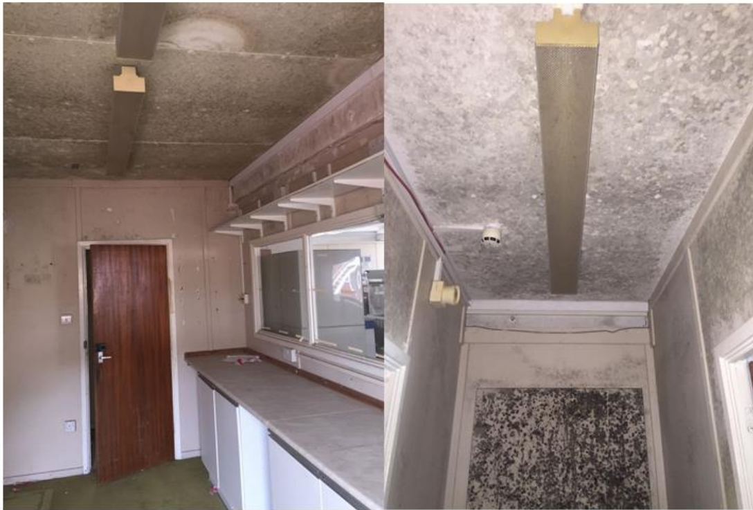
Figure 4-1: Two pictures for mouldy room explaining the growth of microorganisms on the walls and ceilings. This table shown in the left picture was used to install the two bioaerosol samplers.
