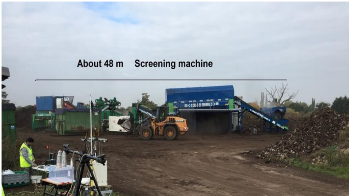
Figure 6-2: Illustrate how the Screening machine can be considered as a line source, where the machine length up to about 48 meters and the emission are emitted from all parts of the screening machine.
