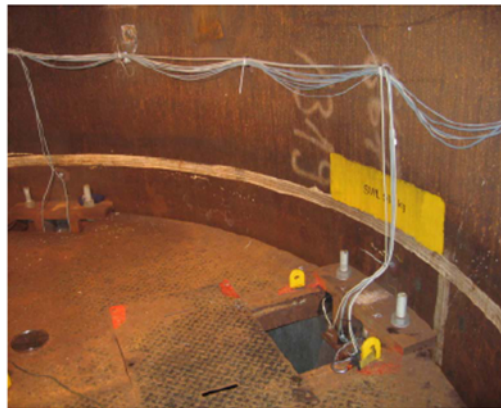
Figure 2-17: Monitoring of corrosion [126]
