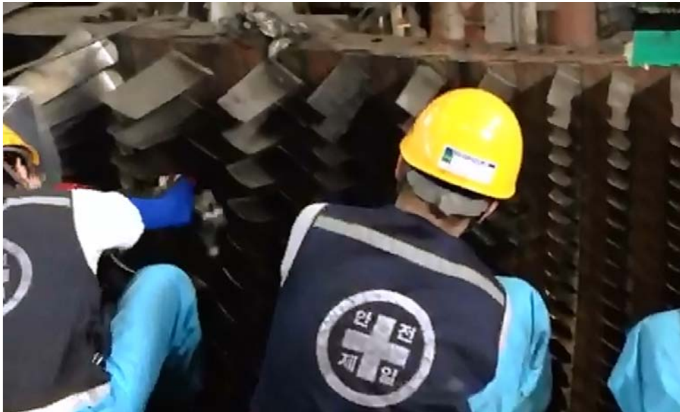
Figure 2-10: Hand cleaning compressor blades (Courtesy of R-MC Power Recovery Ltd)
