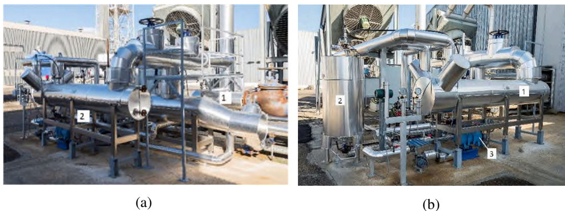
Fig. 4. HC pilot plant at PSA-CIEMAT, exchange circuit: (a) steam generator (1) and surface condenser (2), (b) surface condenser (1), condensate tank (2) and small deposit under the surface condenser (3).
