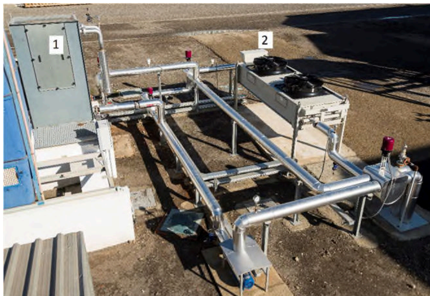
Fig. 5. Cooling circuit in the HC pilot plant at PSA-CIEMAT. WCT (1) and ACHE (2)
