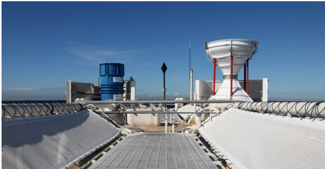
Figure 22: HydroAir VRT-2 prototype installed on Oceanlinx OWC Platform, Australia 2010.
