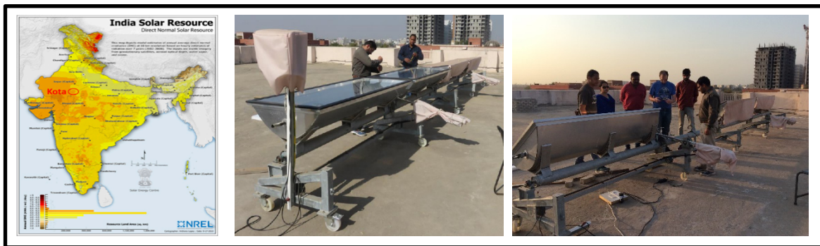
FIGURE 5. Testing location at Kota University showing DNI map [3] and images during installation
