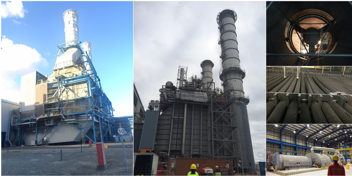
Fig. 2.3 On the left seen two Heat Recovery Steam Generators from two distinct CCPPs. On the right from the top: gas turbine exhaust, superheater tube banks, steam turbine (author's collection)
