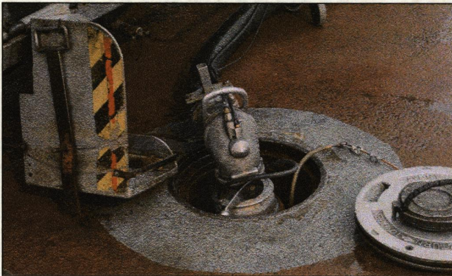
Figure 5-16. A pit where fuel is taken for refuelling. (Photo by Michael Bracha, 2002, Linde Gas, Germany)
