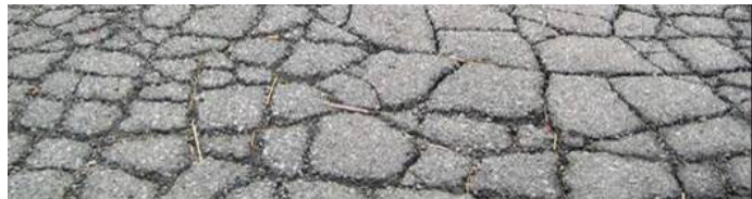
Fig. 3-4 Deteriorated road segment
