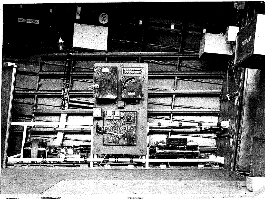
Fig.21. Invertor station with maintenance panels removed.
