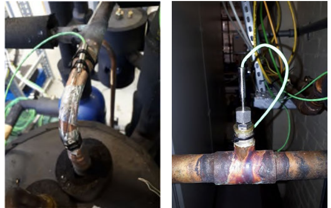
Figure 5: NARROW THERMOCOUPLE (Ø0.75MM) FOR SURFACE MEASUREMENT BEFORE BEING COVERED WITH PIPE LAGGING (LEFT) THERMOCOUPLE INSERTED WITHIN THE PIPE (RIGHT).
