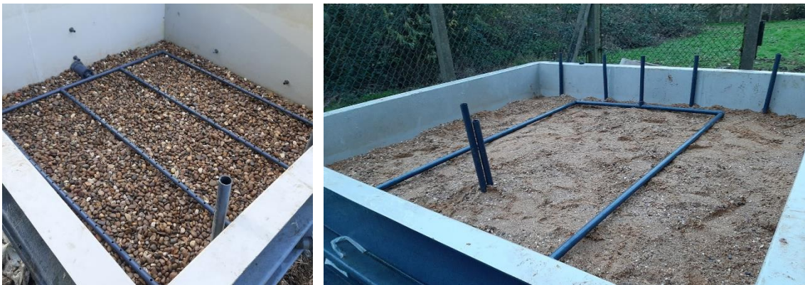
Figure 5.1: Construction stages of the VF wetland a) Drainage layer and collection pipes b) Treatment layer and distribution pipes
