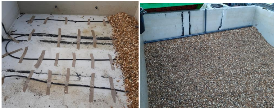
Figure 5.2: Construction stages of the AHF wetland a) Aeration piping and collection area, b) Treatment bed and distribution pipe
