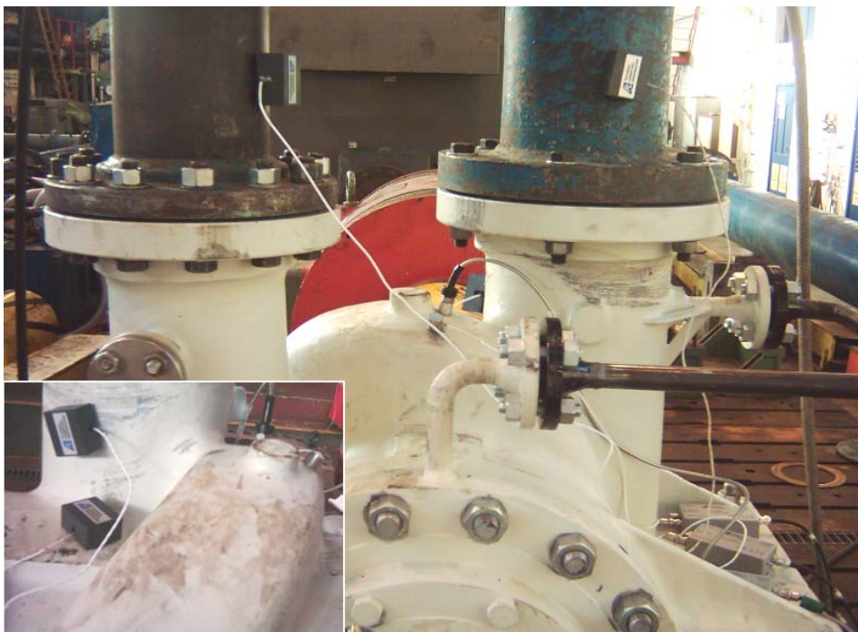
Figure 1 60KW centrifugal pump which underwent performance and NPSH tests showing AE sensor locations
