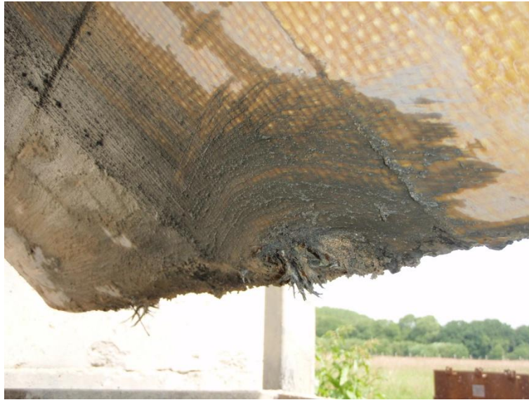
Figure 5-15 Damage to underside of hull C after firing
