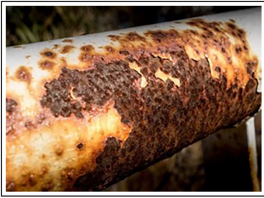
Figure 4. Corrosion in a pipeline and metal skin. 62
