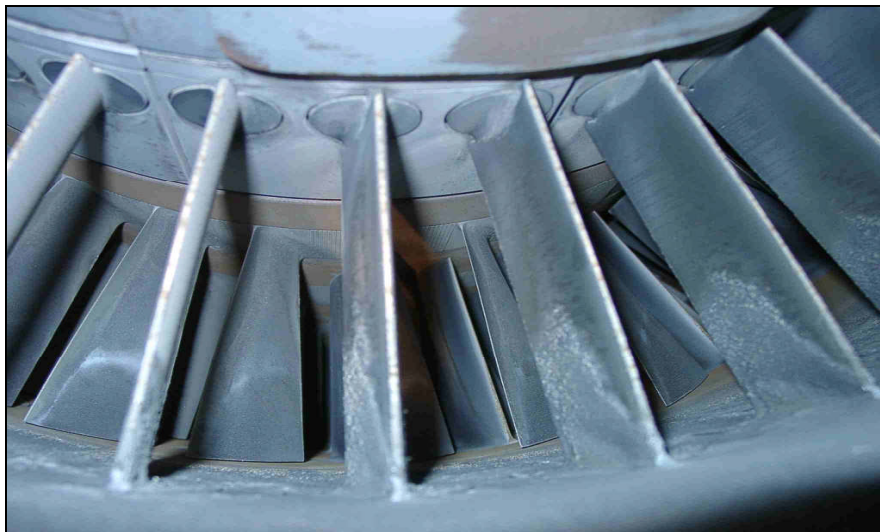
Figure 2-6 The hydrocarbon deposit in compressor IGV and blades (Sulzer type 3, Nafora oil field)
