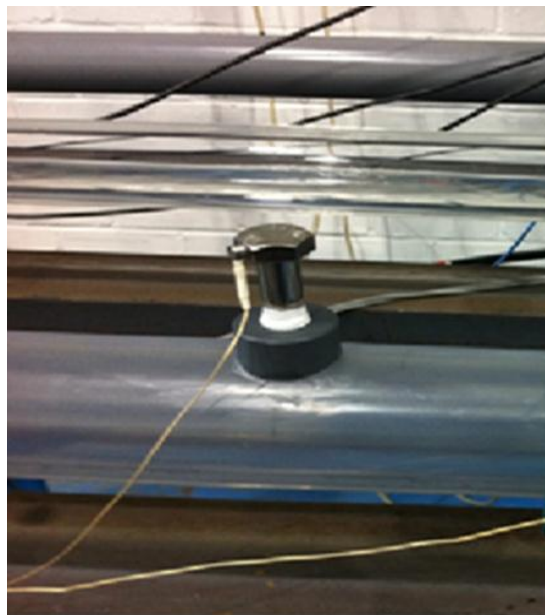
Figure 6-20 M12 waveguide and AE Pico sensor installation for two phase flow regime recognition
