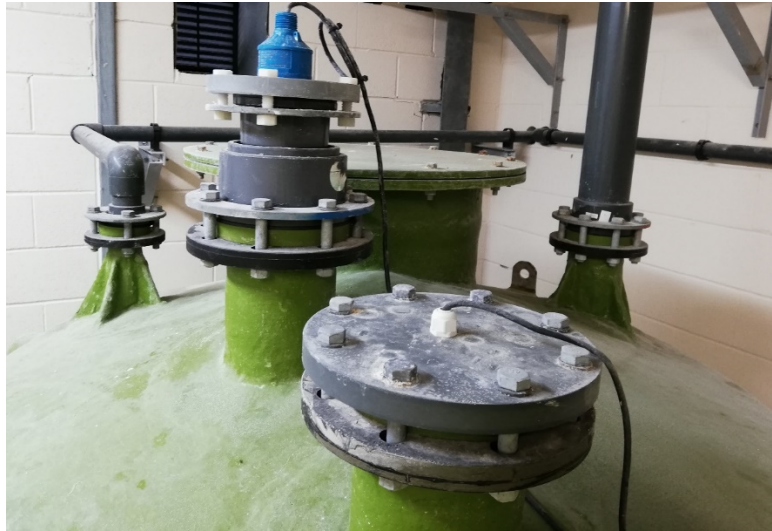
Figure 3-6. Electronic level sensors for hypochlorite tanks.
