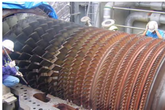
Figure 5 Fouled rotor blades of heavy-duty engine compressor
