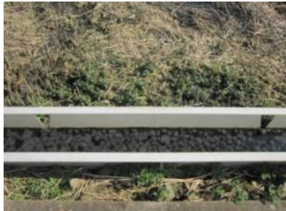
Image 2. V-notches of the inlet channel.
