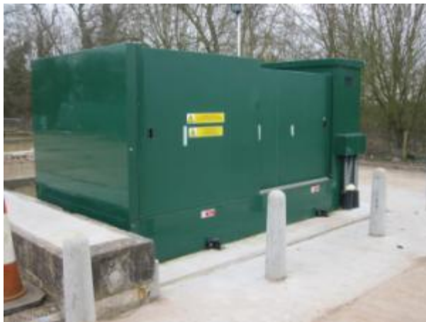
Image 8. New ferric sulphate dosing tank.
