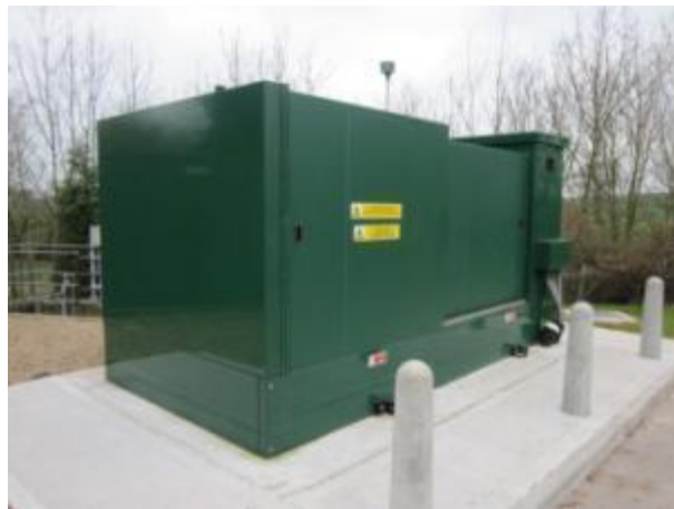
Image 5. New Ferric sulphate dosing tank.
