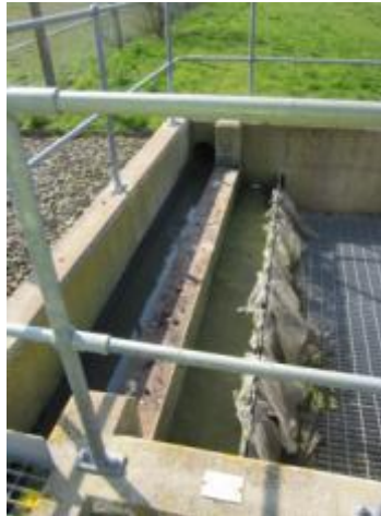
Image 7. Copa sac screening system for storm water.
