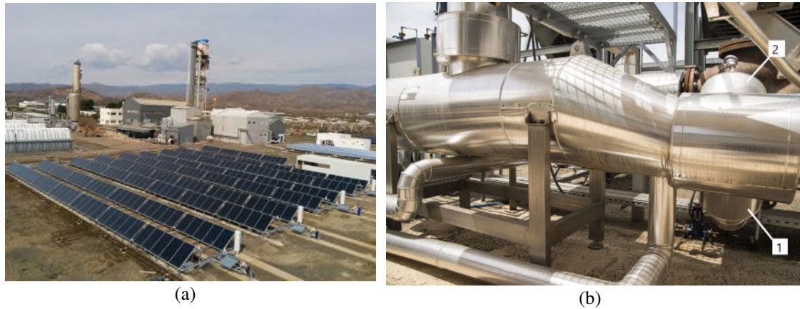
Fig. 3. HC pilot plant at PSA-CIEMAT: a) flat-plate collectors of the heating circuit, b) steam generator: hot water inlet (1) and outlet (2).
