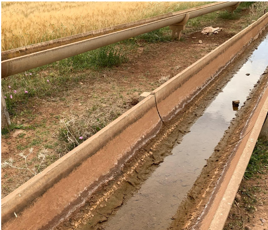
Figure 4-2 Irrigation system consisting of elevated concrete canals arranged in a hierarchical structure.
