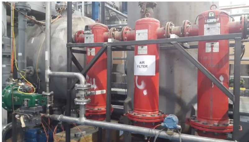
Figure B-2 Air supply filtering and metering system of the three phase rig
