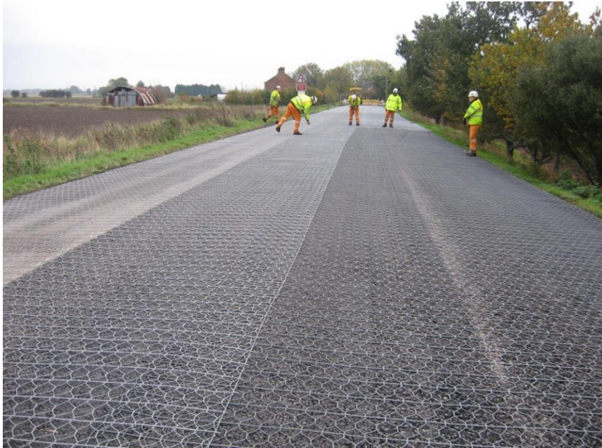
Figure 5-13: Installation of steel reinforcing grid on Lincolnshire highway (Photo: Lincolnshire County Council)
