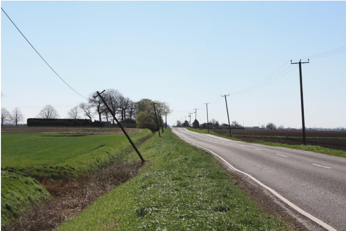
Figure 2-3: A section of the A1011, Bates Drove, Norfolk, showing leaning telecommunications pylon (left) and undulating road surface due to soil shrinkage.
