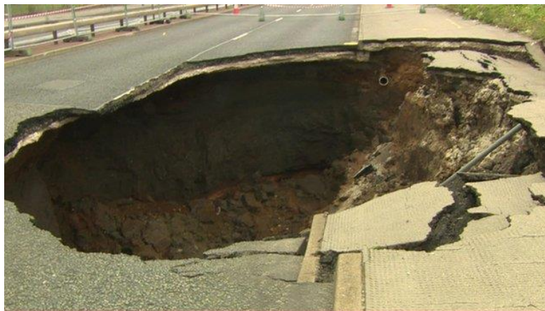
Figure 6-4: Cavitation causing extensive damage to the Mancunian Way, Manchester as a result of a burst water main (source: BBC, 2015)
