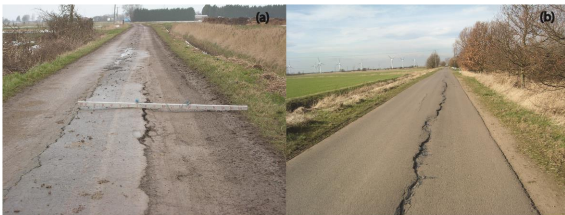
Figure 5-4: Examples of Lincolnshire road subsidence; (a) Childers Lane, Spalding; (b) Cowbridge Road, nr Bicker (Photos: Lincolnshire County Council)
