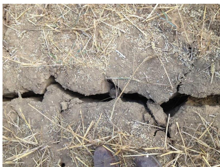
Figure 3-2: Horizontal shrinkage crack in clay soil, Northamptonshire, UK (Photo: O. Pritchard)
