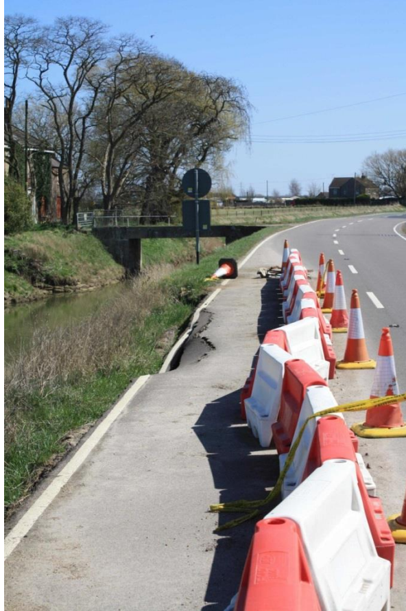
Figure 5-14: Road embankment instability, B1165 Ravens Bank, Lincolnshire
