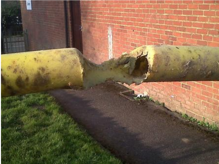
Figure 6-14: Polyethylene gas main damaged by high pressure erosional (sand & water) slurry (Photo: Northern Gas Networks)
