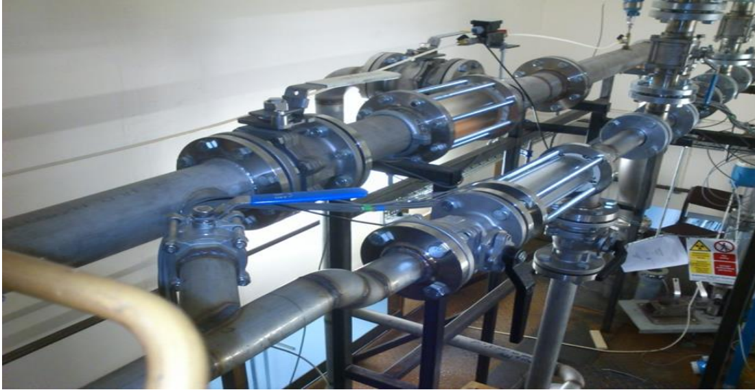
Figure 3-12 Intermittent absorber coupled with 4” pipeline-riser system
