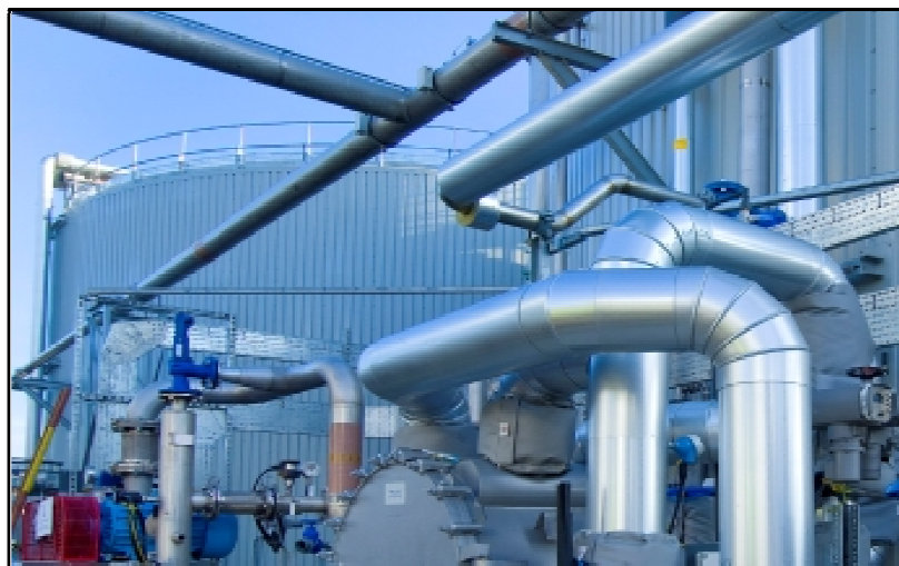
Figure 3.6. Full scale anaerobic digesters, Esholt STW, UK.
