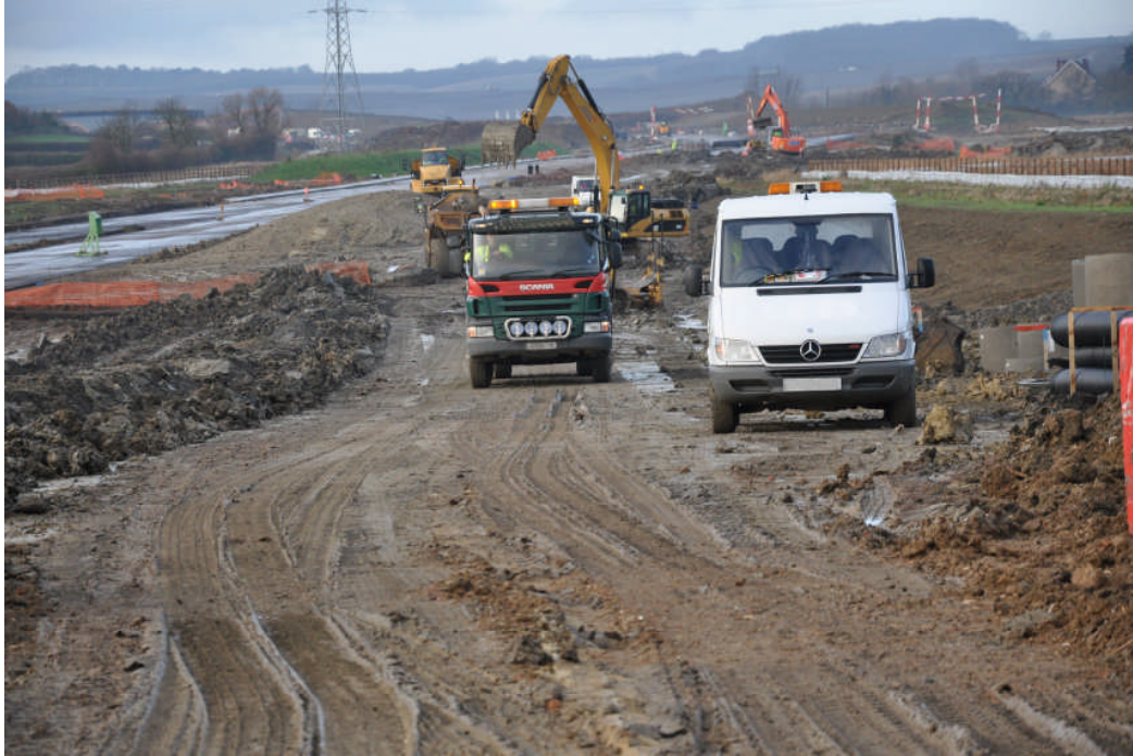
Figure 34 – Typical construction truck road used by 8x4 construction truck's to deliver aggregate.
