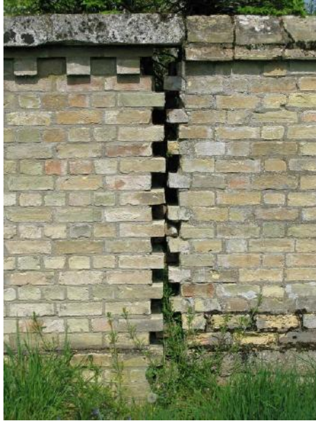
Figure 1 The effects of severe clay-related movement on brickwork. (Wimpole, Cambs. S. Hallett)
