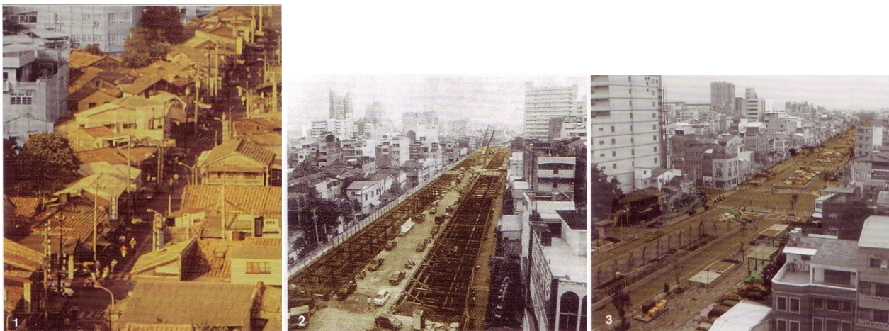
Figure 3.6. The before, in progress and after photo of Haiian road's expansion construction.
