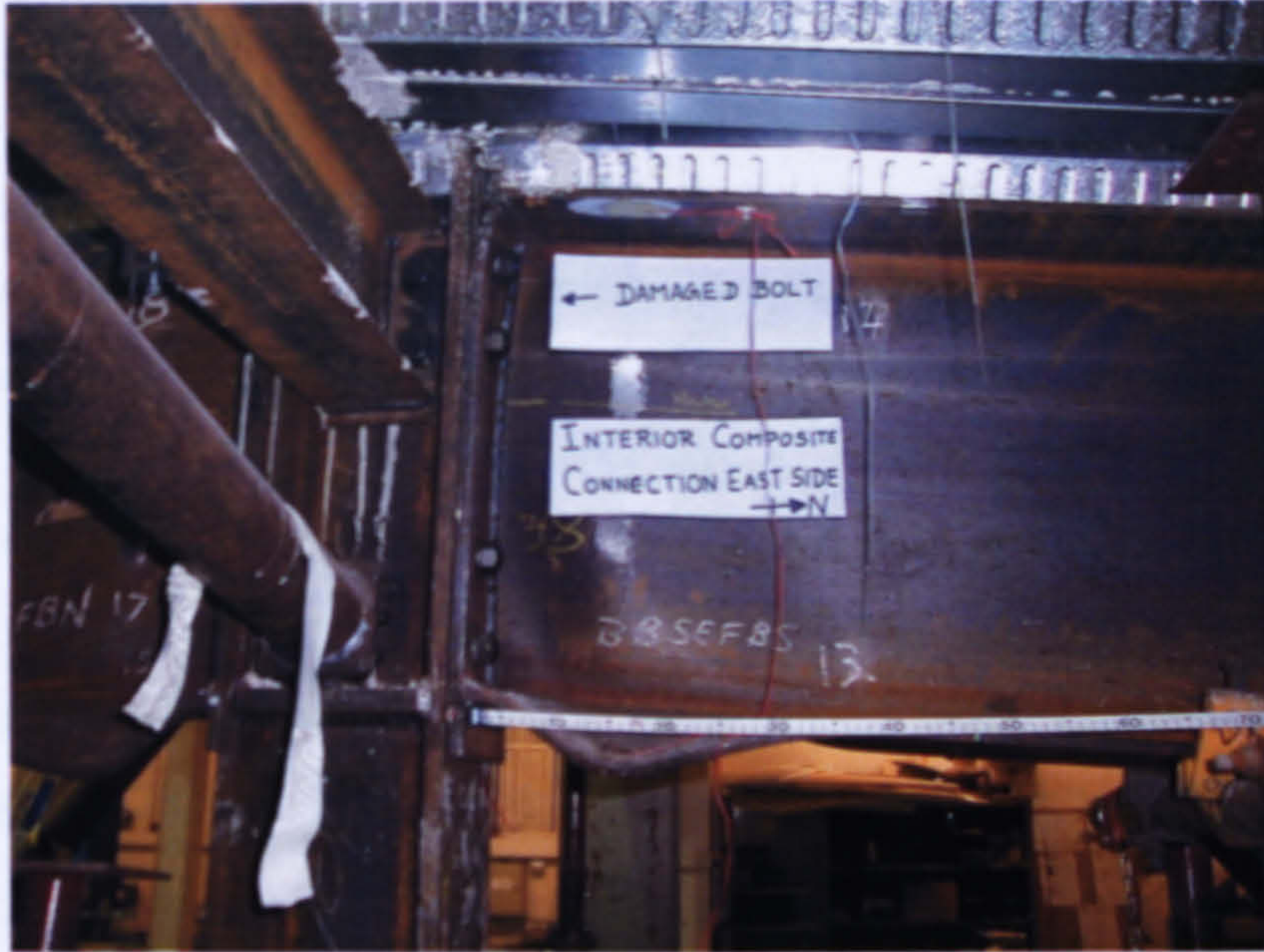
Figure 3-27. Interior composite connection (moment connection side) after test frame failure
