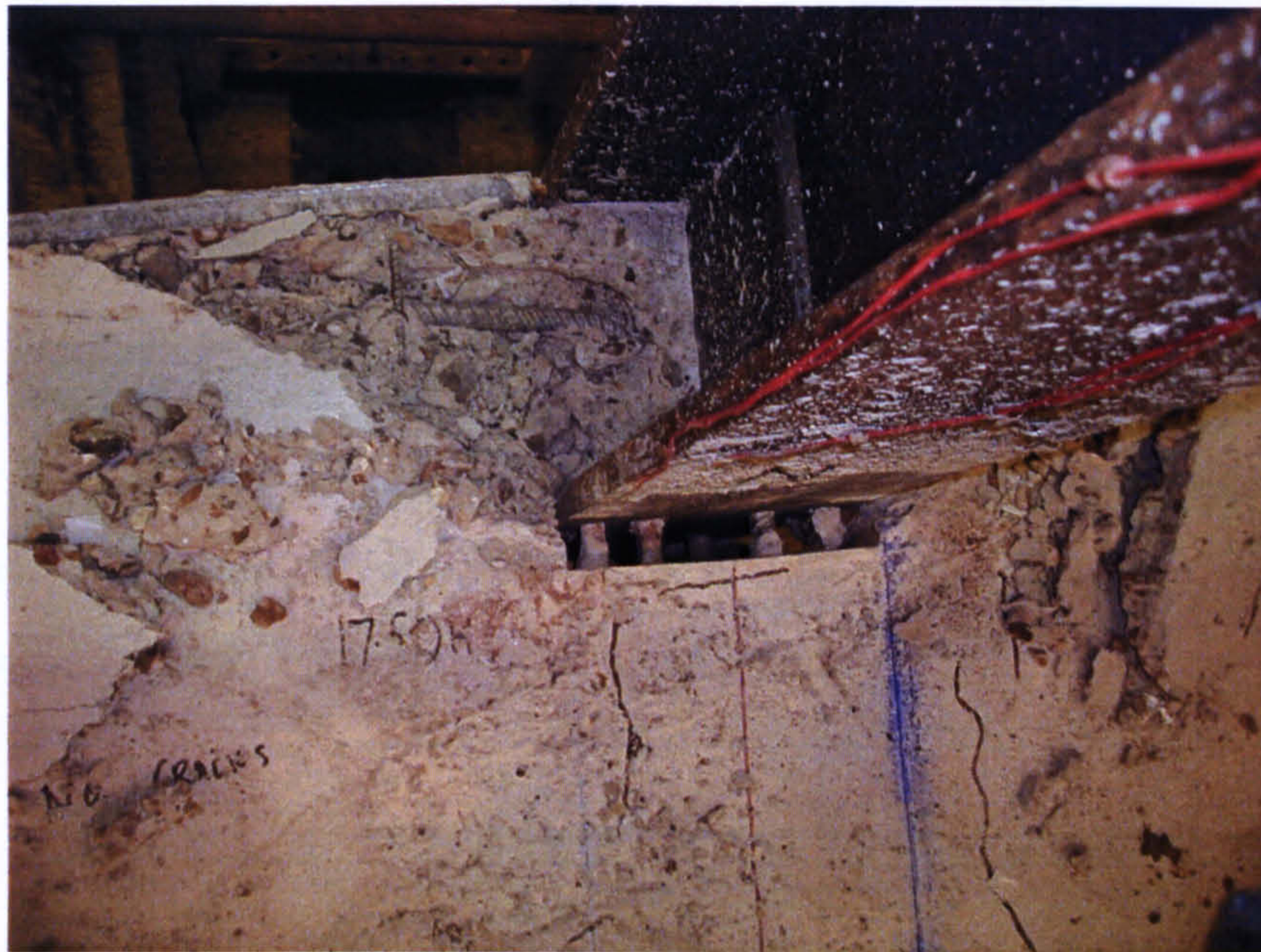
Figure 3-24. Cracks observation in the exterior composite connection side
