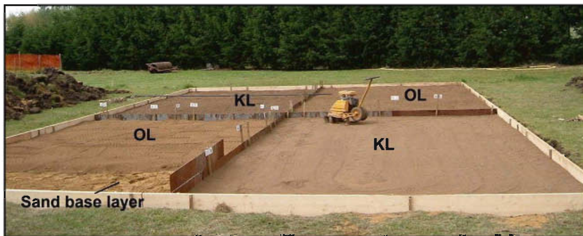
Figure 5.1 Trial plots during construction May 2005. Two soils Kettering Loam (KL) and Ongar Loam (OL) were laid in opposing corners enabling 10 individual plots for each soil. Rolling was undertaken in 10 rolled strips 1.3 m wide (from left to right / right to left in this picture) covering both soil types.
