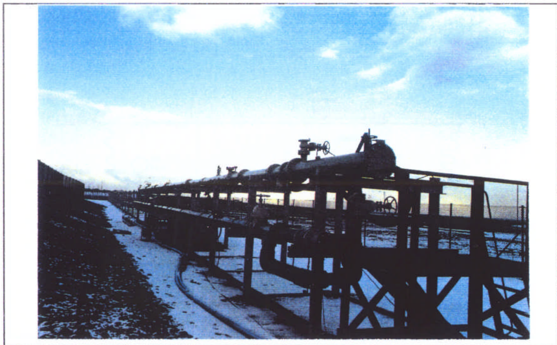
Figure 6.4 Overview of the entire facility
