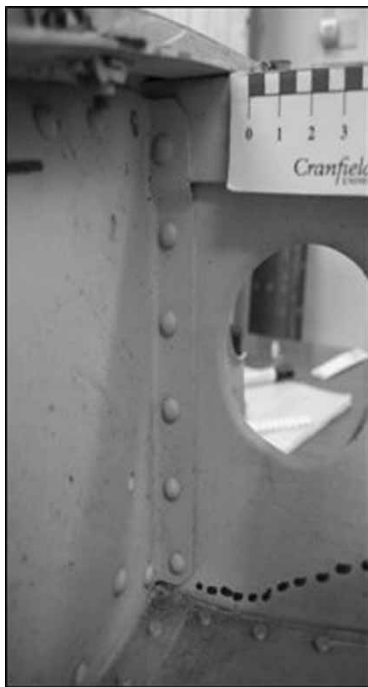
Fig. 13 A lack of intersection joint collapse is a common feature observed during a water impact, as the intersection between STN370A and V0 orientated normal to the water surface demonstrates
