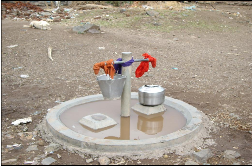
Plate 10: Leaking Taps, with flooded aprons
