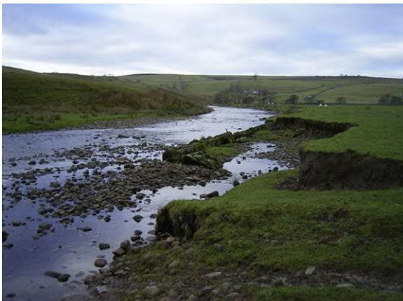
River bank erosion upper Eden
