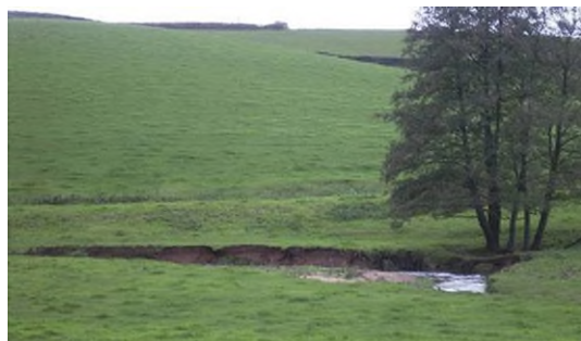
River bank erosion
