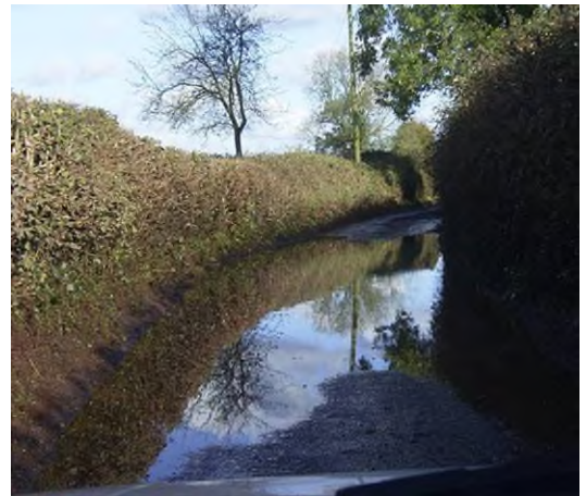
Local road flooding
