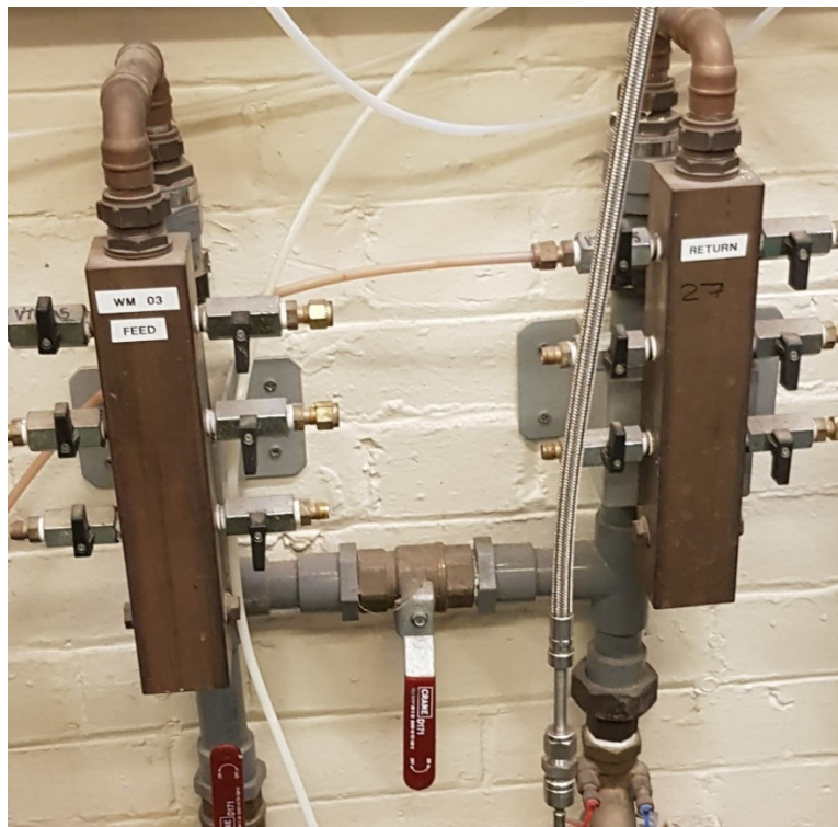
Figure 5-4 Copper pipes in the system attached to the furnaces, via multi-port system which are nickel plated brass fittings
