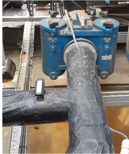
Figure 5-3 Steel filter housing
