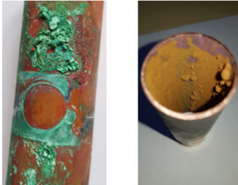
Figure 5-5 Corrosion on Cu tubes(a) on outer surface (b) iron oxide internally
