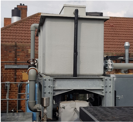
Figure 5-2 PVC storage tank
