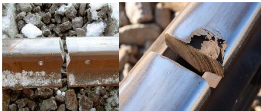
Fig. 3. Sample Rail track breaks.
