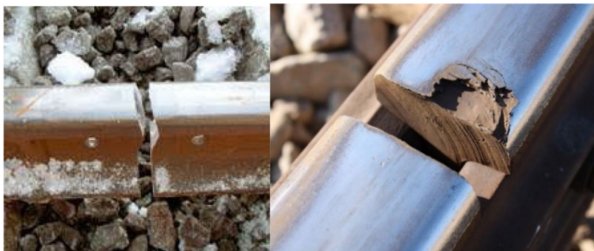
Fig. 3. Sample Rail track breaks.
