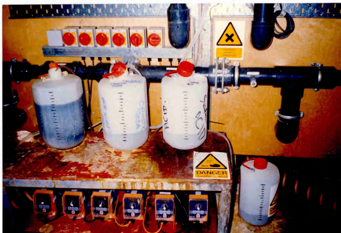
Figure 4.10. Photograph showing pre-treatment chemicals and dosing pumps.
